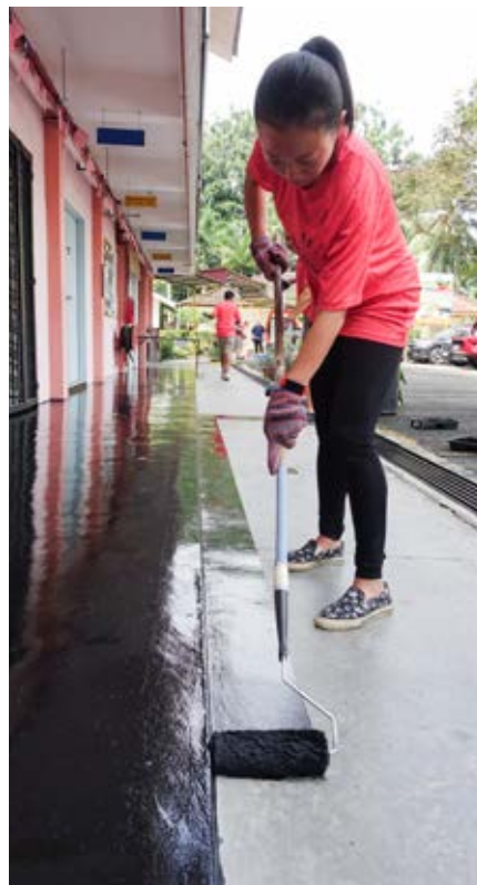
A fresh coat of paint to spruce up the corridors of SK Bukit Lanjan.
